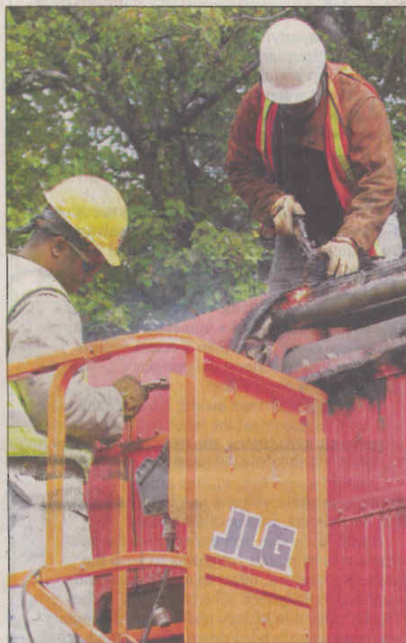
Above: On Monday afternoon, Winter Environmental employees work on demolishing the Pullman railcar on Mill Street near Marietta Square. Inset: The Pullman car as it was on Mill Street. Left: From left, Tivone Harrell and Lee Gottins, employees for Winter Environmental, work on demolishing the railcar on Mill Street. Below: Gottins cuts the railcar.
